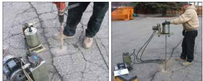
Prior to completing subgrade soil compaction and reinforcement with polymers, a DCP test is performed. A hole is drilled through the concrete or asphalt surface (left). Then an automated hammer (right) drives a steel cone into the soil using a metered rod. Blow counts recorded indicate the relative density of the soil.
